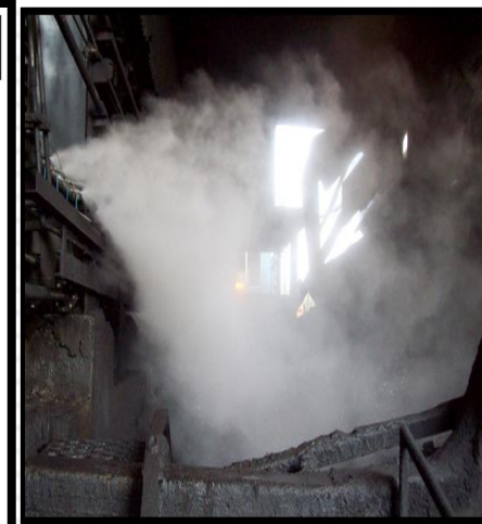
Dry fog system at Wagon Tippler
